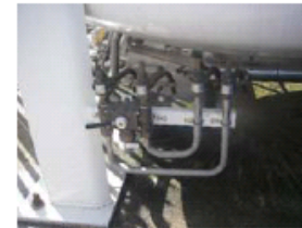
Typical tank relief valves
