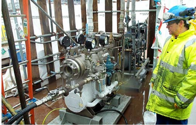
'The ZugiBeast' at the RPLG Refrigeration Unit, at BP, Grangemouth.
