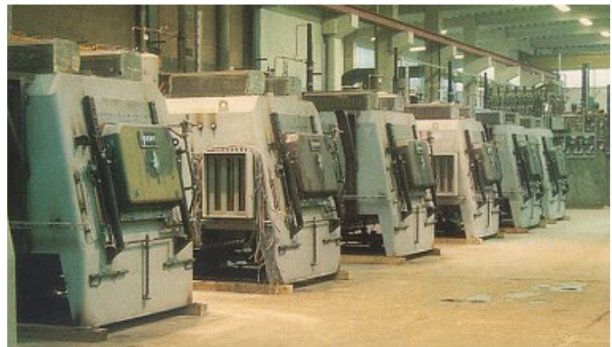
Figure 3. Sealed quench furnaces
